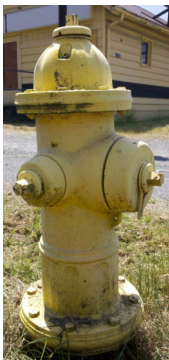
This is an example of a properly maintained hydrant.
